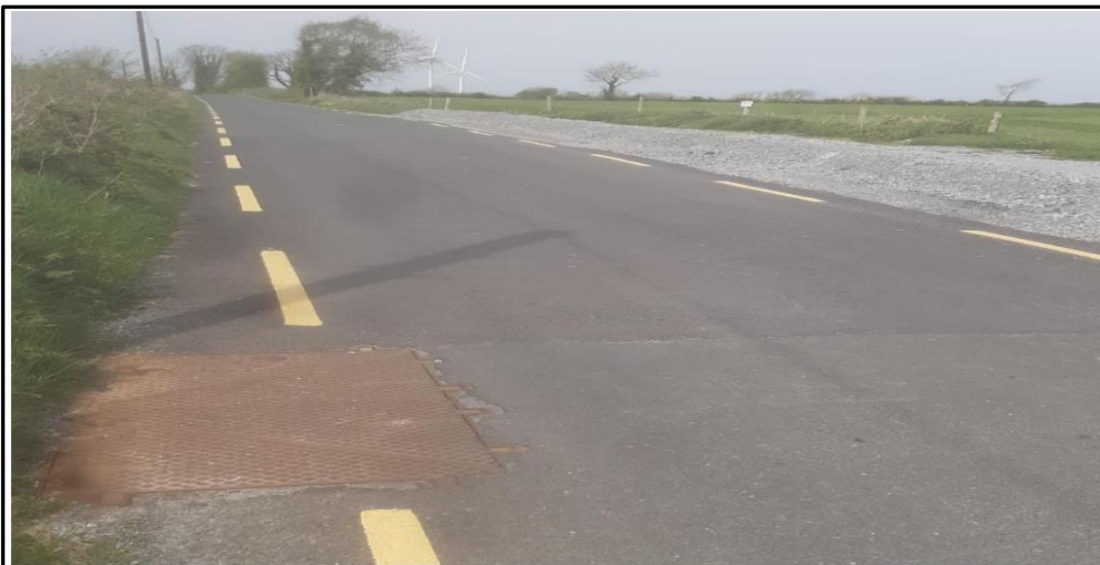
Image 6.12: Example of a Reinstated Road Over a Joint Bay (Darker Asphalt) with the C2 Chamber Cover Visible
